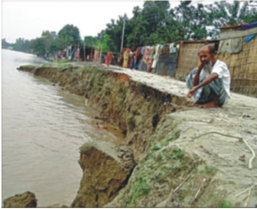
Figure:7 River erosion
